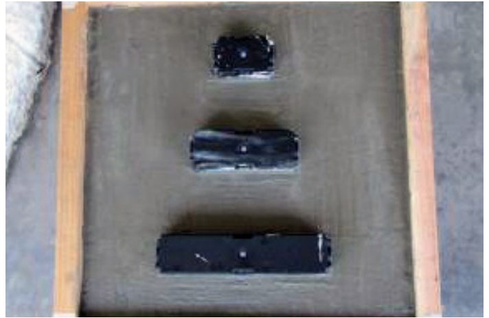
STEP 1 Pour the RIS into concrete wall, making front surface of tray flush with form.
